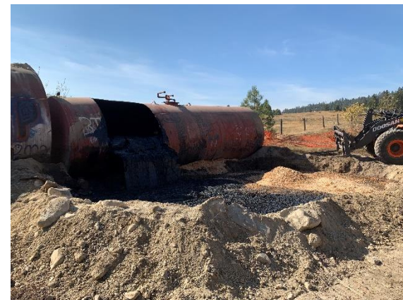
Tank #13 drains in solidification pit
